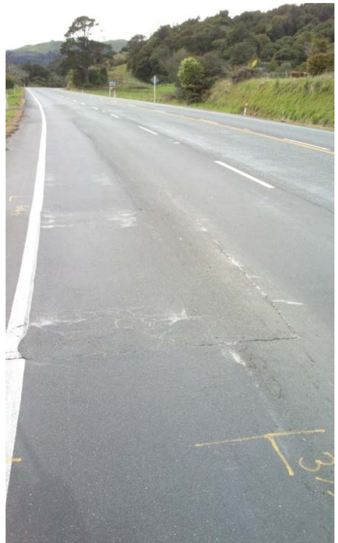
FIGURE 6. PHOTO OF PAVEMENT DISTRESS AT HELCOR SITE
